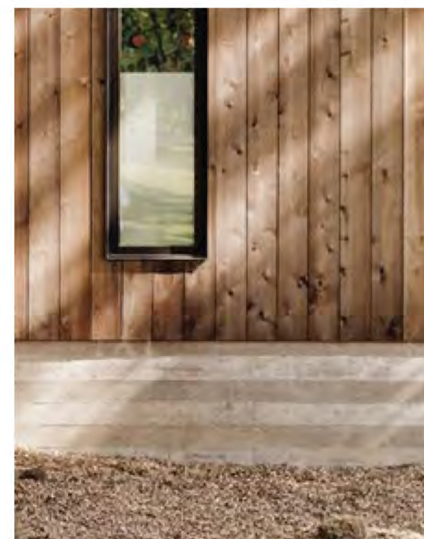
Concrete foundation. Exposed surfaces of concrete are formed with narrow boards leaving a horizontal imprint of the cladding texture. Clear seal finish
