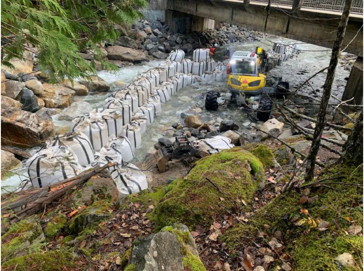
Photo 1 - Spider Excavator Installing Site isolation and Diversion in the aptly named 'Crazy Creek'
