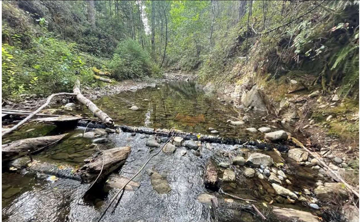
Photo No. 3 Date: 19 September 2023 Looking Towards: West Location: Upstream of Mackie Road Dam
