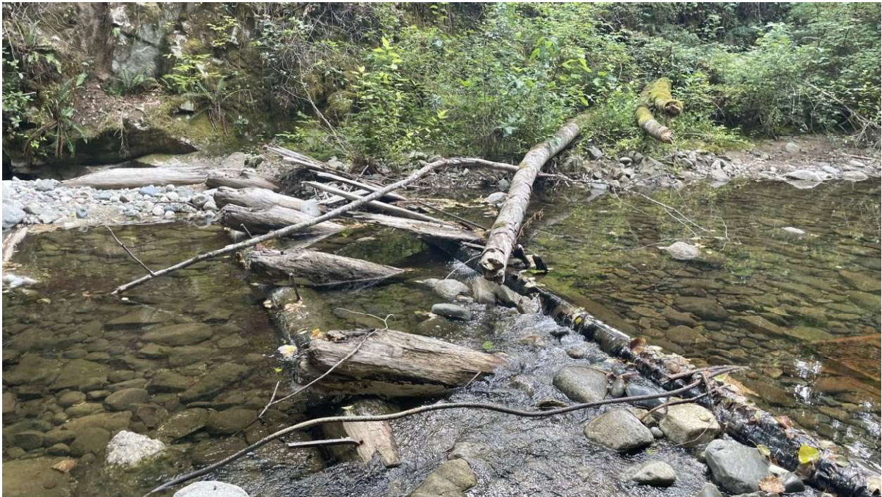
Photo 8 Vegetation built up on remnants of wooden flashboards on right side of upstream channel & miscellaneous debris.
