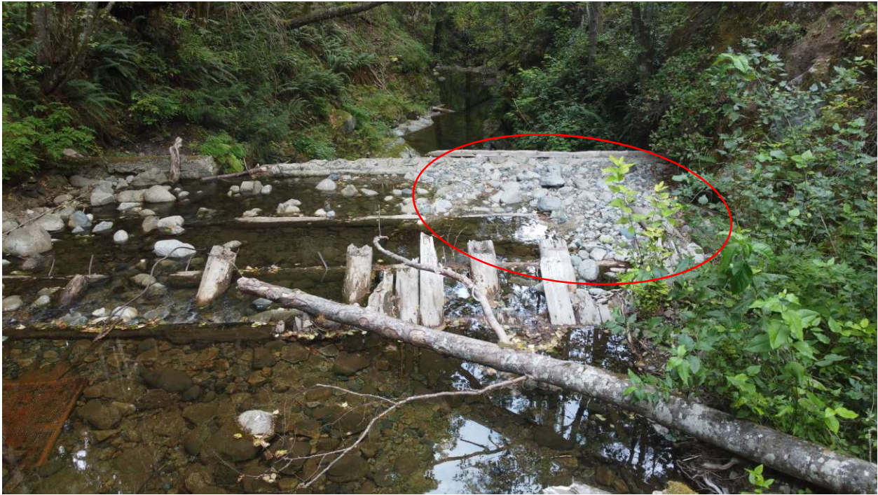
Photo 3 Top of dam with debris buildup on right side, looking northeast (downstream).
