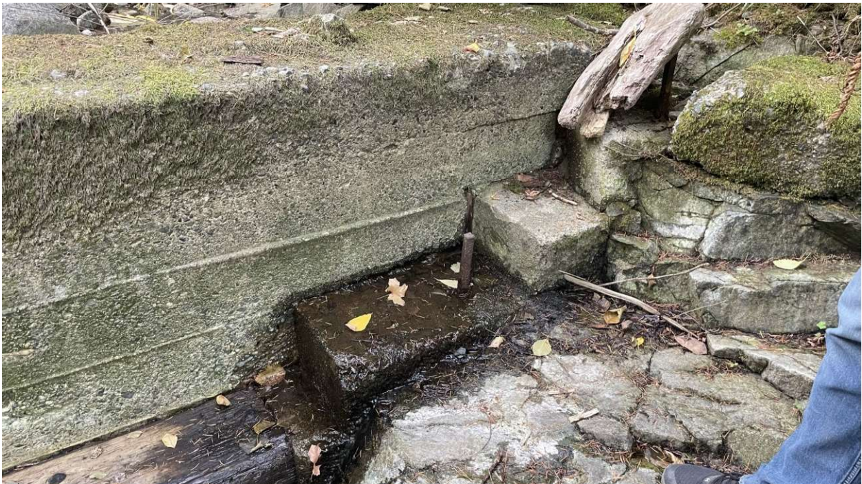
Photo 6 Seepage underneath left concrete abutment.
