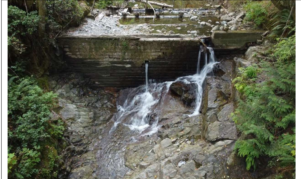
Photo No. 1 Date: 19 September 2023 Looking Towards: West Location: Mackie Road Dam Description: Looking at Mackie Road Dam during the low flow period.
