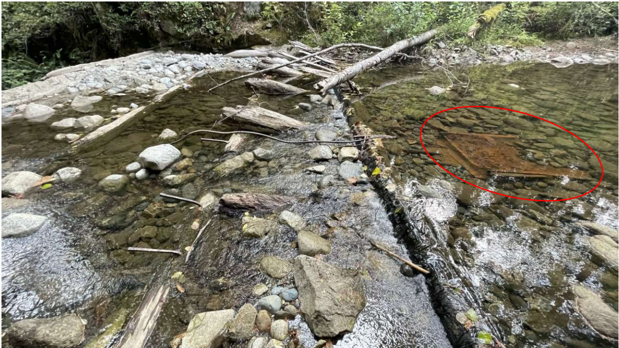
Photo 2 Low-Level metal intake grate and remnants of wooden flashboards, looking east (from left side of dam).
