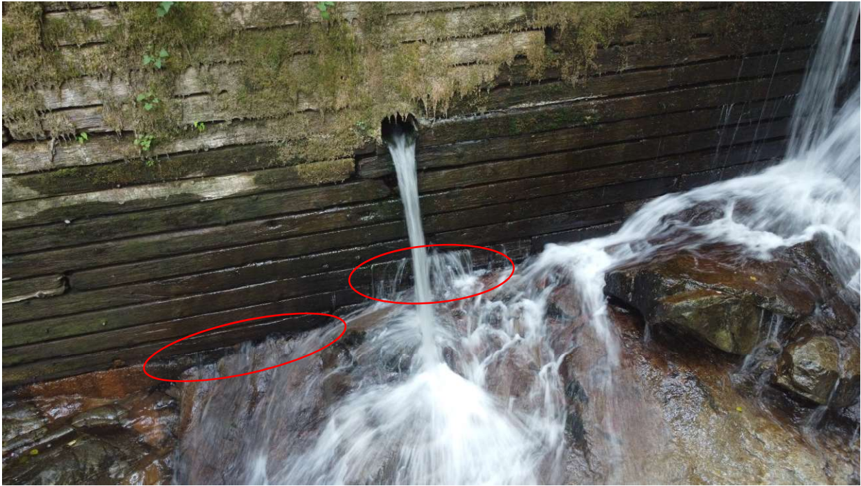
Photo 7 Major seepage at toe of downstream face.
