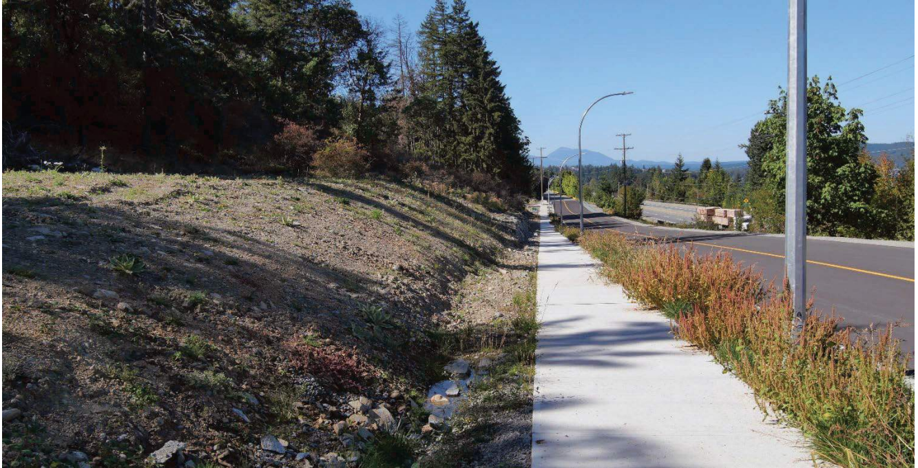
Figure 2.2.c: Slope above sidewalk along Farrell Road
