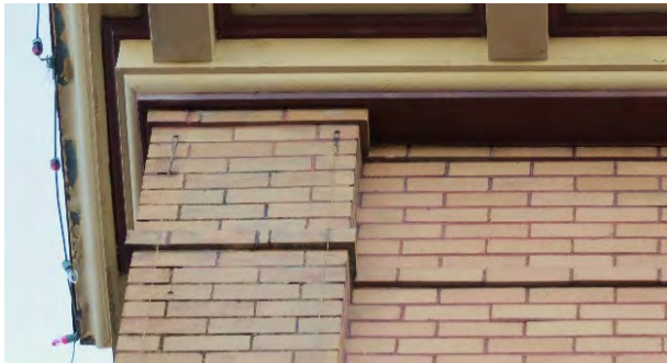
Column expression full height at both corners; two horizontal single brick raised bands;
