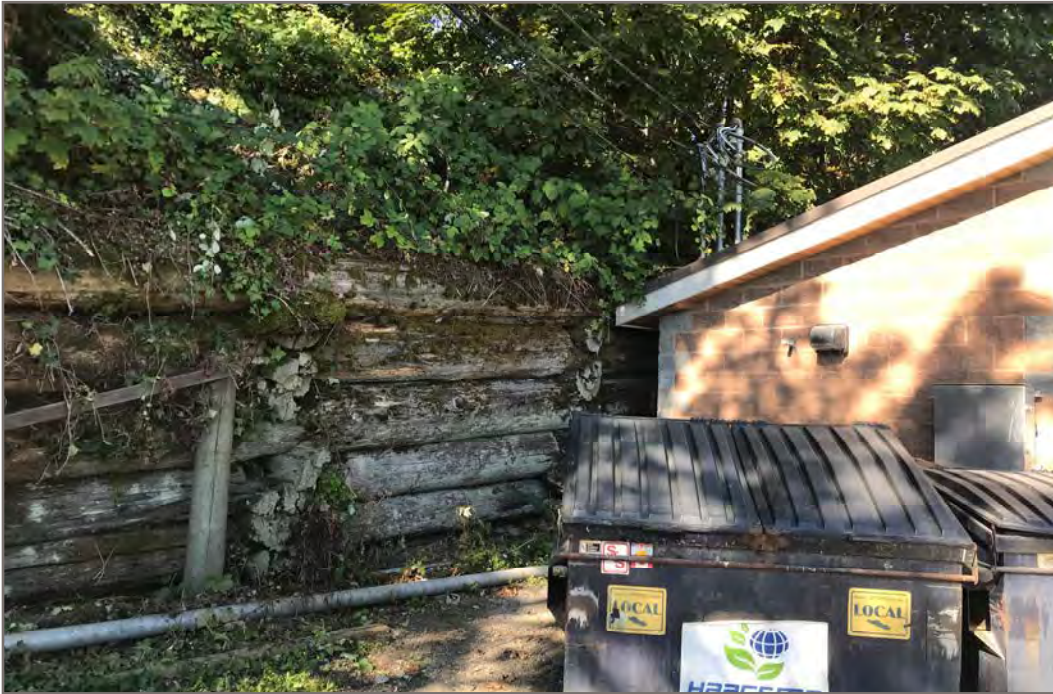
Photo 1: Failing Log Retaining Wall behind existing Power Building
