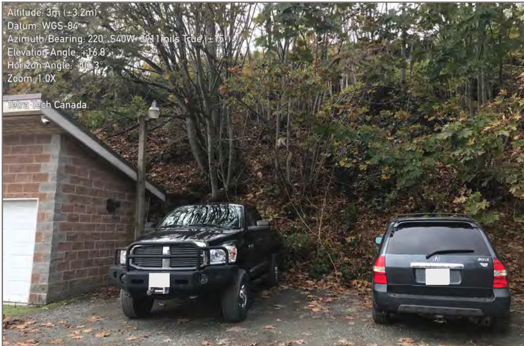
Photo 3: Slope Northwest of Failing Retaining Wall
