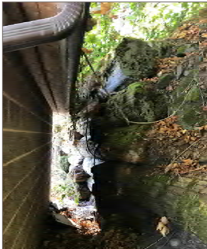
Photo 2: Failing Log Retaining Wall, Looking behind the existing Power Building
