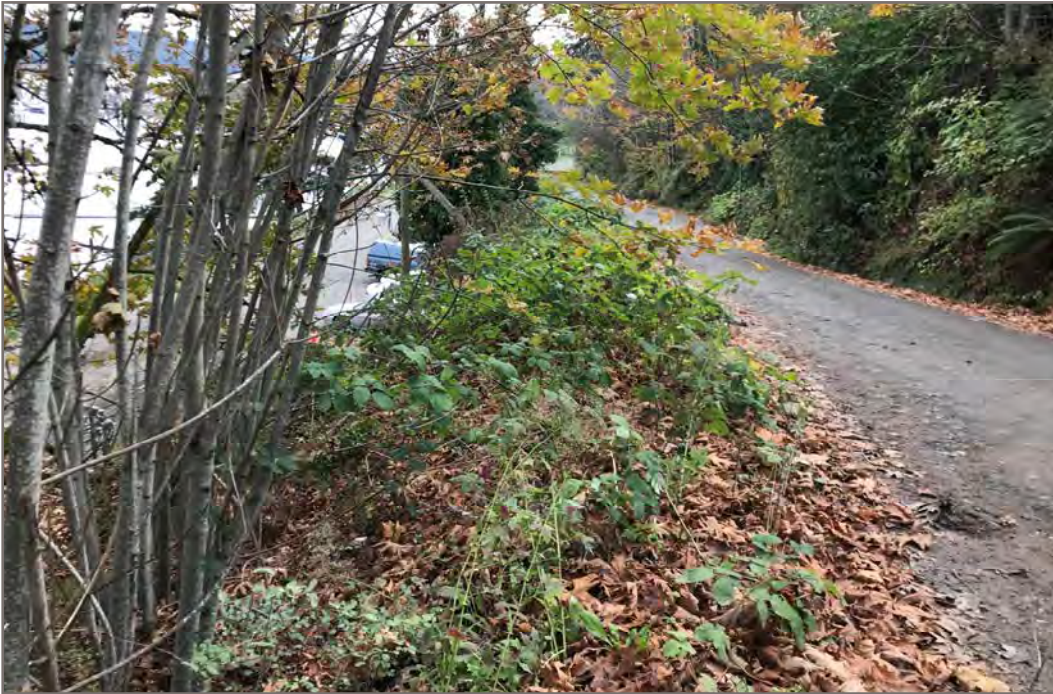
Photo 5: Oyster Bay Drive, above Failing Retaining Wall, Looking Southeast
