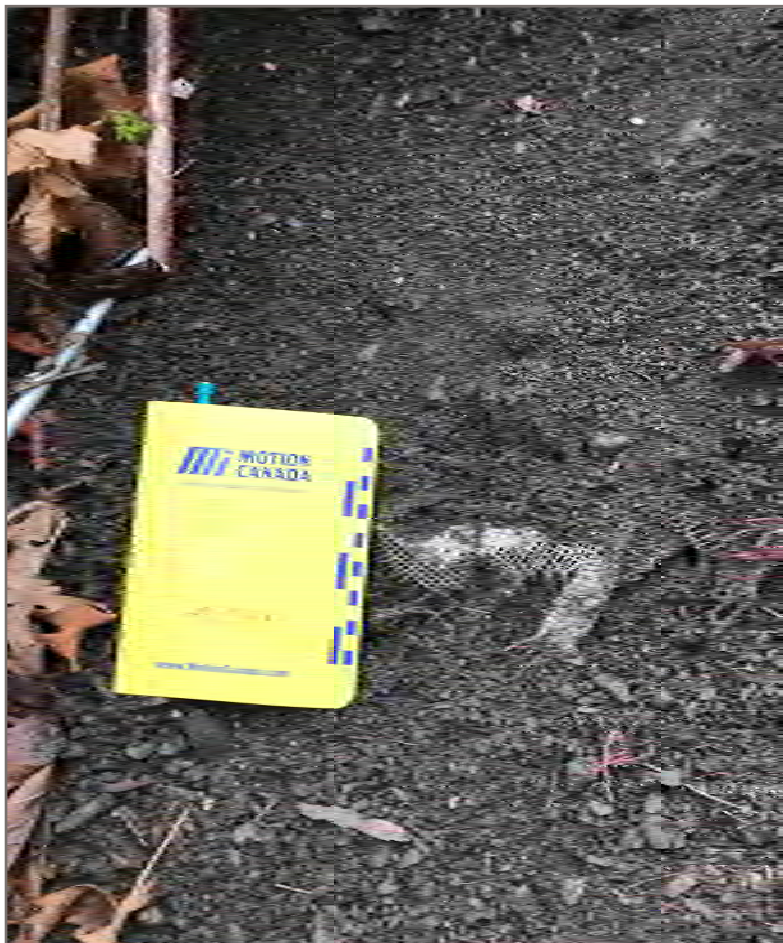
Photo 4: Erosion Protection Matting / Geotextile on Slope Northwest of Failing Retaining
